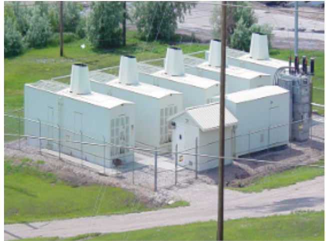
Figure 05-3. Ben French Diesel Generators
