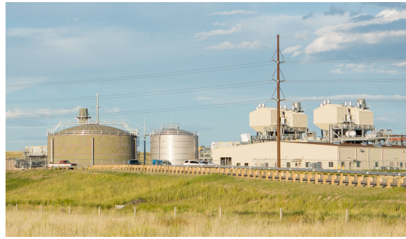
Figure 05-8. Cheyenne Prairie Generating Station Combined Cycle CT
