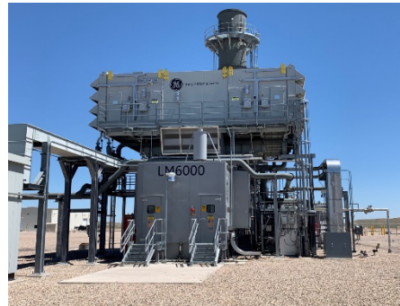
Figure 05-2. Cheyenne Prairie Generating Station Simple Cycle CT
